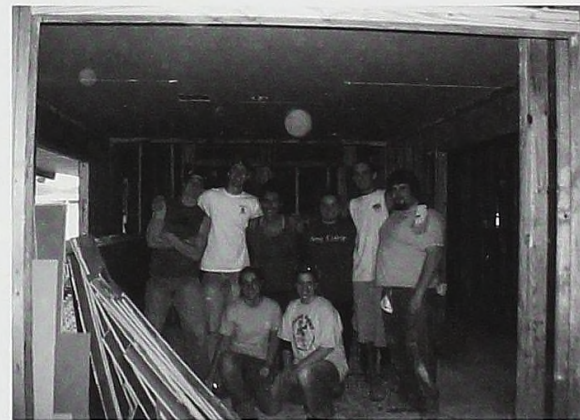
Alma College Students spend Winter Break 2007 in Louisiana assisting the National Relief Network. "The Best Dry Walling Crew" takes a break for the picture below. Photo Courtesy of Chris Francis '09
