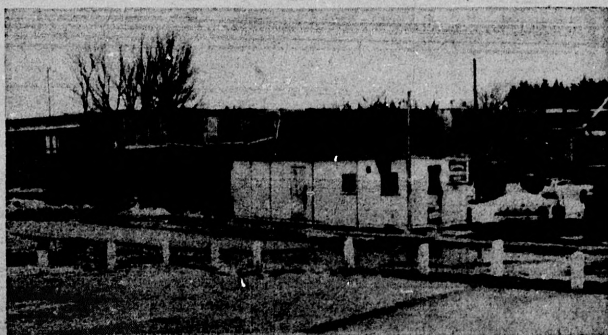
Work is progressing rapidly on the science building. With the west wing enclosed in plastic, workmen have a wind-free area in which to finish the interior. This past week saw the be-
