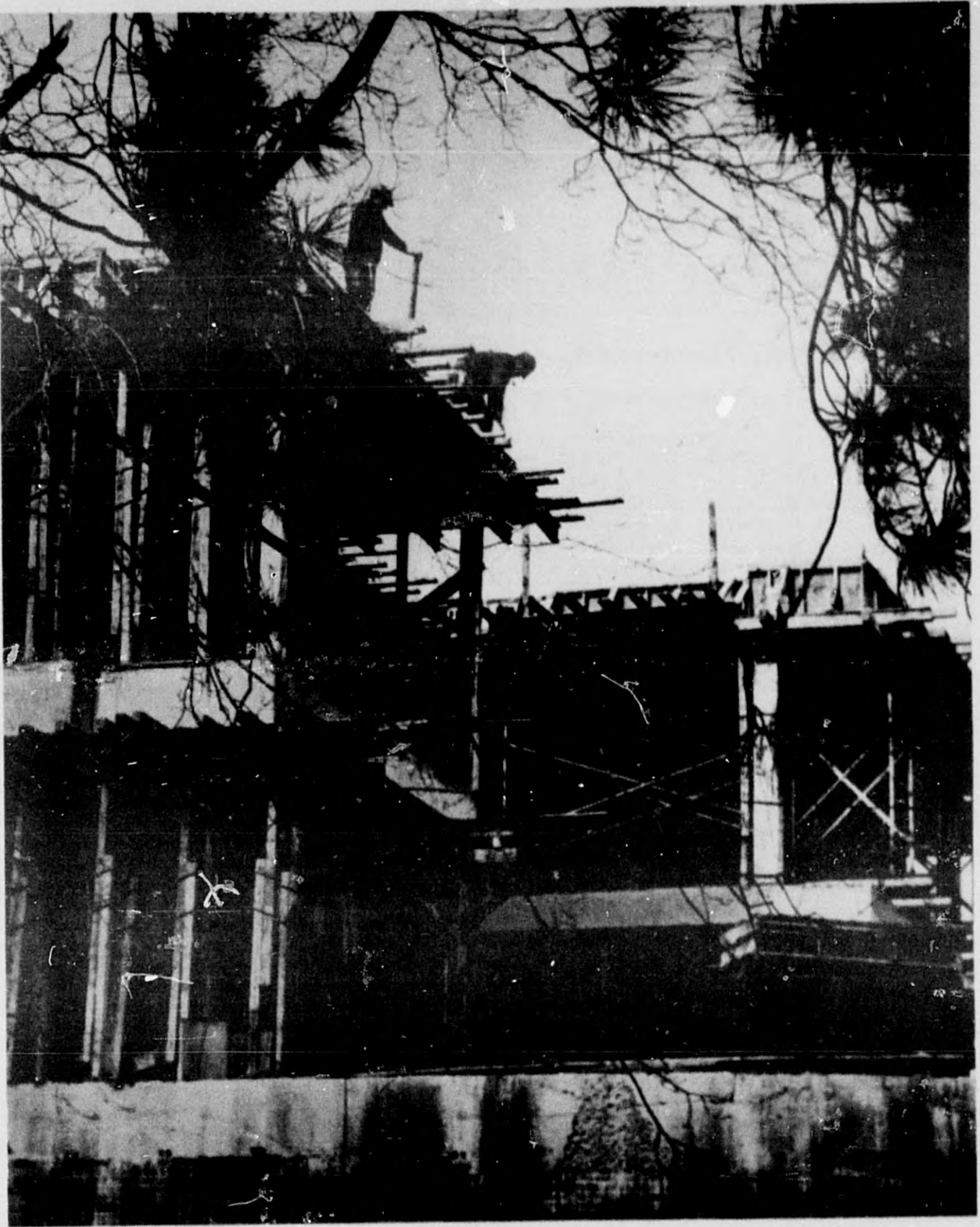
Framed by branches of a nearby pine, workmen prepare forms for the roof of Alma College's new four-story Academic Center. Milder than usual weather this winter has helped to keep construction on schedule, and it is anticipated that the building will be ready for use by the end of this year. The Academic Center will include 61 faculty offices and 28 classrooms, two observation-classroom-testing facilities, a computer laboratory center and three psychology laboratories with adjacent experimentation rooms. The new building, the seventeenth major construction project at Alma within the past two decades, is located near the site of Old Main, a classroom-office building that was destroyed by fire in March of 1969.
