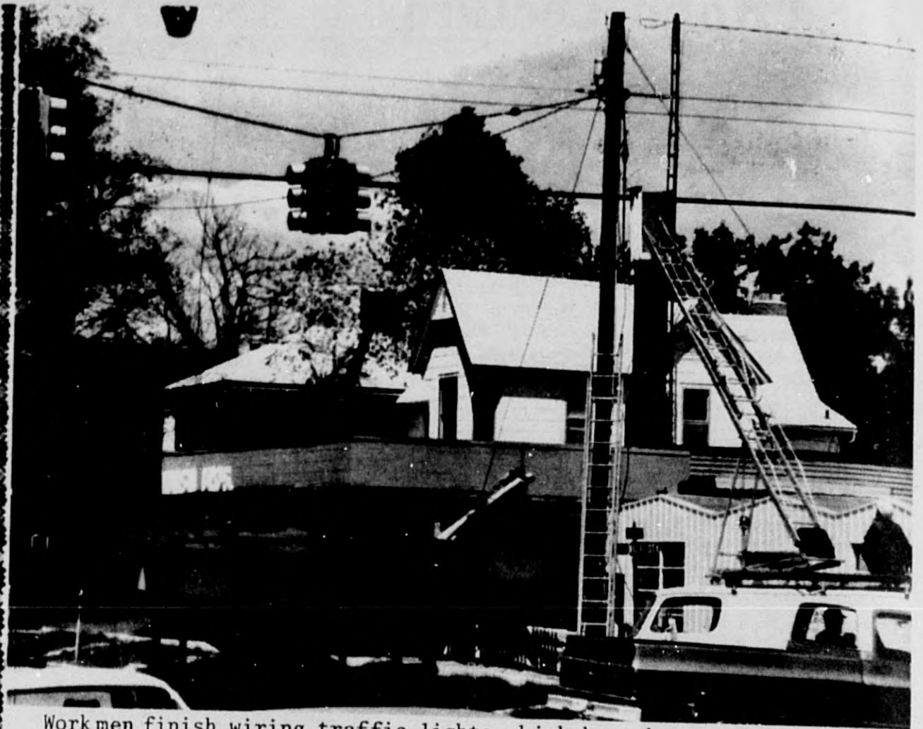
Workmen finish wiring traffic lights which have been put up at the corner of Woodworth and Center Streets to control rush hour traffic. The lights will blink for another week so motorists will become accustomed to them.
